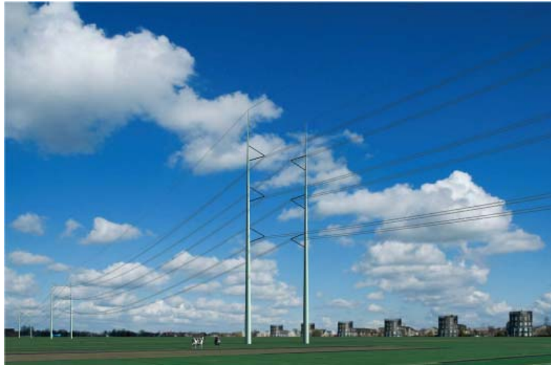
Figure 6-13 Wintrack tower design for reduced magnetic field levels under 400 kV lines (source TenneT)
