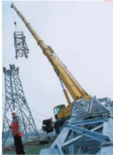
Figure 4-2 Assembling of preassembled steel segments by the use of a mobile crane (source: E.ON Netz website)
