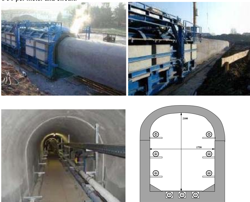
Figure 75 Infrastructure tunnel, system Dupré, Speyer; above: construction works, below left: installation of equipment in the tunnel, below right: schematic drawing of tunnel cross section with three UGC circuits
