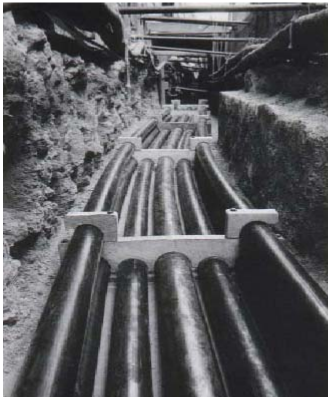
Figure 69 Laterally cooled UGC in Vienna with four cooling pipes (two between cables and two above outer cables)
