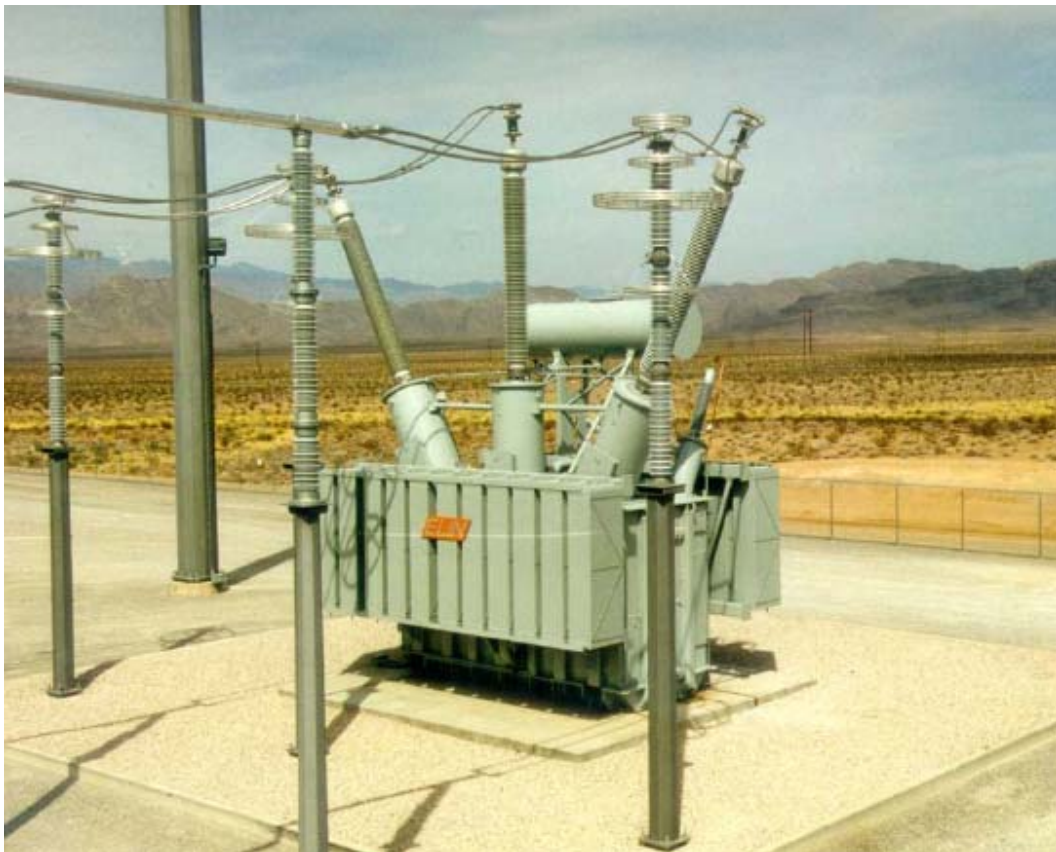
Figure 4-12 400 kV, 160 MVA shunt reactor for reactive power compensation (source: [CIGRE_B1.07 2006])
