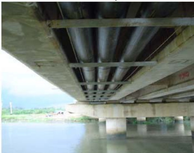
Figure 6-5 Bridge used as river crossing for cables; source: [Cova 2008]
