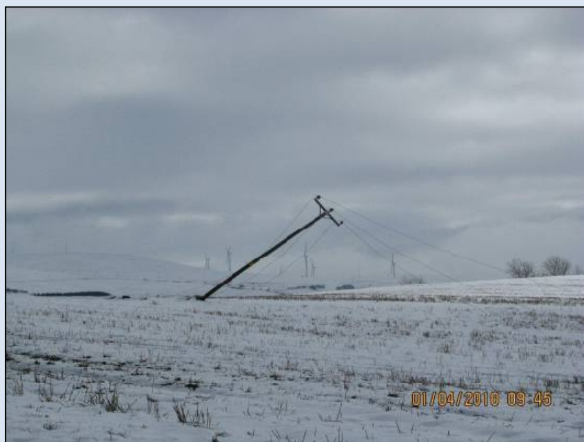
Figure 5-5 Example of damage during the March ice storm. Image courtesy of NIE.
