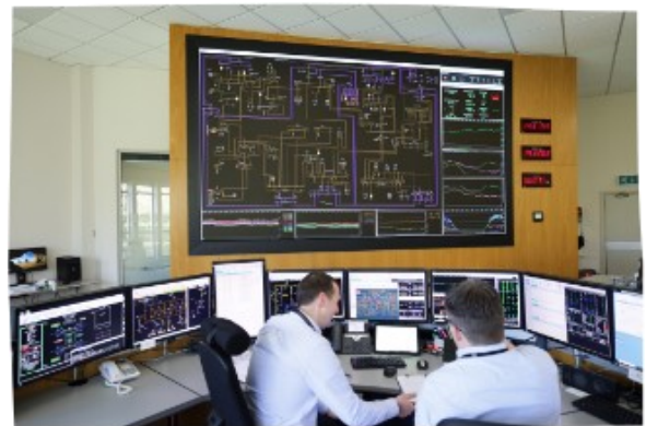
SONI Control Room
